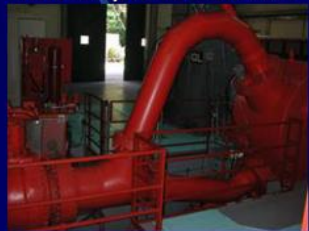
Pelton turbine in a SHP station of Dominica
