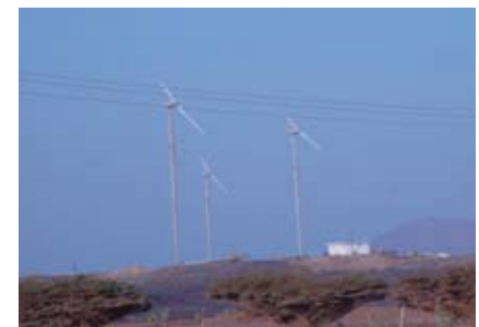
Assad wind farm (Photo courtesy of UNDP)
